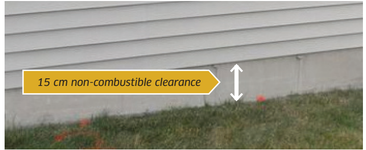
HAZARD FACTOR 7: GROUND TO SIDING CLEARANCE
